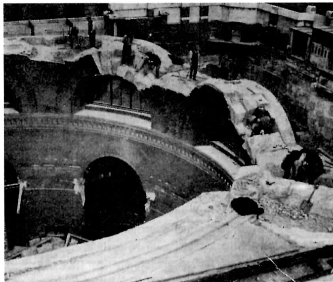
Gandy's prophesy came true when the Bank was demolished in 1925, as pictured by The Times on 1st May.
